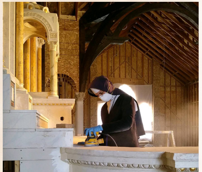
Armed with a dust mask and electric sander, Sister Mary Cecilia works on the altar at Saint Joseph's in Olathe, Colorado. The Sisters have been doing detail work in the new church.
