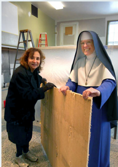
All hands on deck! Rev. Mother helps out with the kitchen renovation work.
