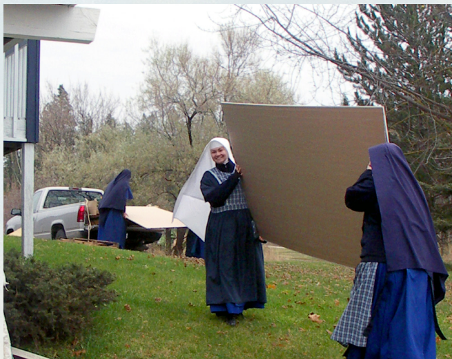
The Sisters at the new Novitiate carry in sheet rock to finish the walls in the basement.
